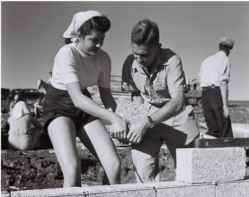
Figure 2: Settlers start building the first concrete block house at Kibbutz Dovrat, 1946 (Kluger Zoltan, Government Press Office. CC BY-NC-SA 2.0). 5
